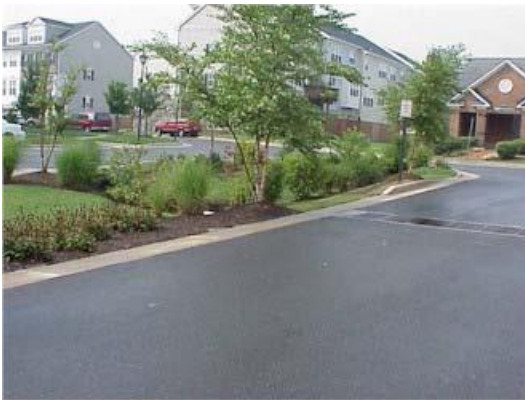
Flow Entrance: Trench Drain
